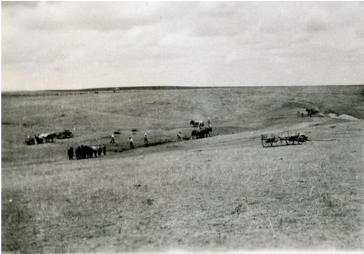
Figure 53. CCC-ID enrollees at work on an unspecified dam site located on the Rosebud Indian Reservation (Rosebud Sioux Tribe). Courtesy of the National Archives (Identifier 12577763).
