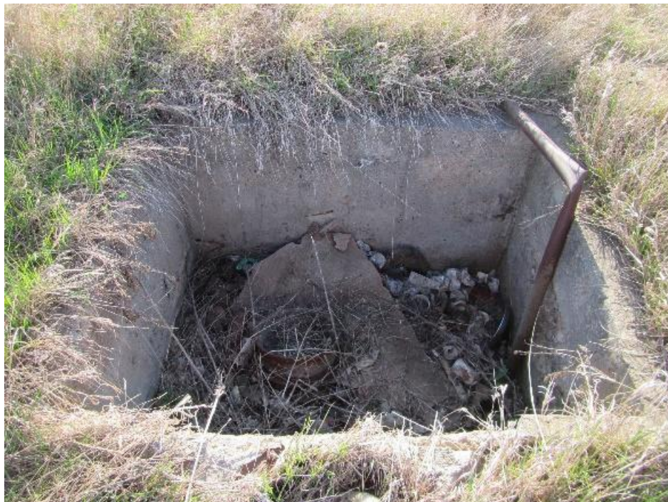
Figure 91. Overview of dilapidated pumphouse, filled with historic and modern trash, Recorded at Site 39CD197, a historic farmstead. 459
