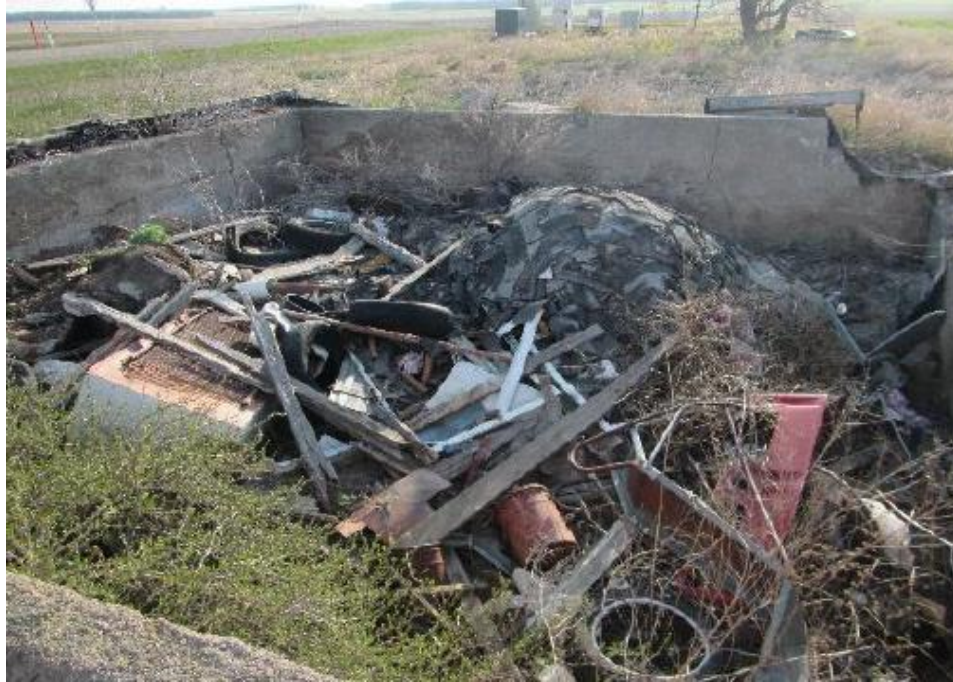
Figure 92 Close-up of dilapidated pumphouse, filled with historic and modern trash, recorded at Site 39CD197, a historic farmstead. From Denekamp and Buhta, “Cultural Resource Evaluation of 176th Street Enhancement Project.”
