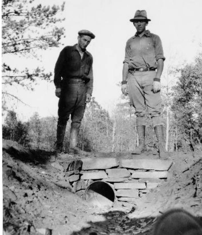
Figure 78. Inlet to 15" culvert constructed by CCC enrollees at Custer Camp F-12. Courtesy of Black Hills National Forest Historical Collection, Leland D. Case Library for Western Historical Studies, BHSU (Identifier BHNF20141180).
