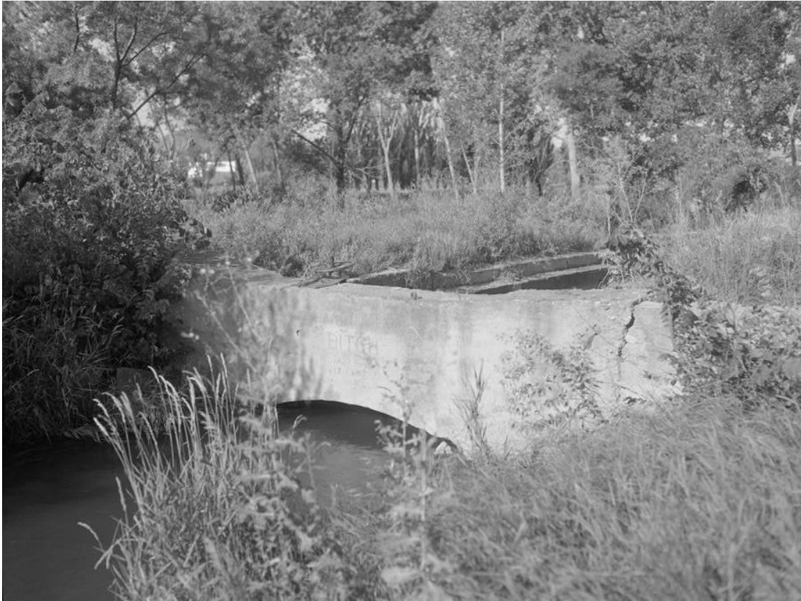
Figure 3. The headgate of the Hawthorne Ditch consists of a concrete wall with a low arch. The side facing downstream reads, “Hawthorne Ditch, Established July 10, 1886.” Courtesy of the Historic American Engineering Record (HAER) (SD,52-RACI.V,2-3).
