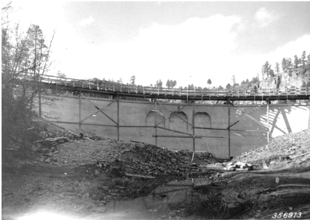
Figure 44. Downstream side of the Victoria Dam, under construction in 1937. Photograph by C. C. Averill. Courtesy of Black Hills National Forest Historical Collection, Leland D. Case Library for Western Historical Studies, BHSU (Identifier BHN20220684).
