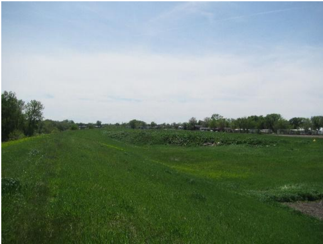
Figure 87. Levee on western bank of the Big Sioux River in North Sioux City, South Dakota.
